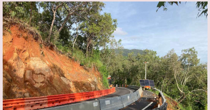
Captain Cook Highway – damaged guardrail (April 2024)
