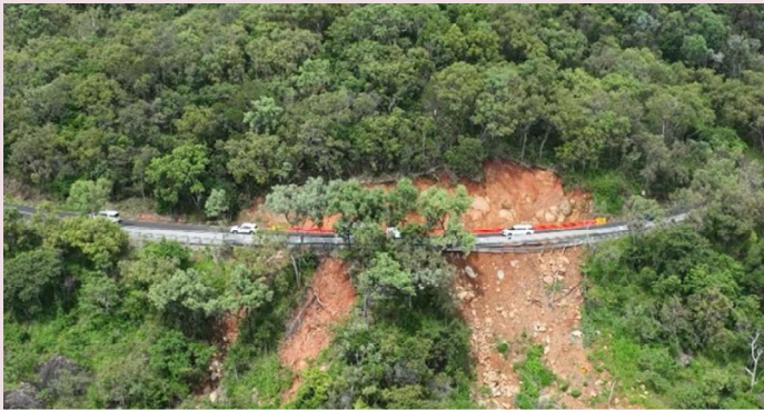
Captain Cook Highway – landslip site (March 2024)
