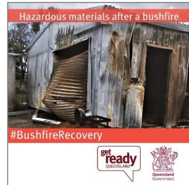
Filename: BushfireRecovery - Hazardous materials after a bushfire
