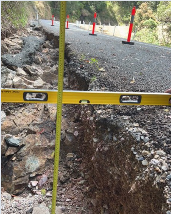
Pine Creek Road – damage from South East Queensland Severe Storms
