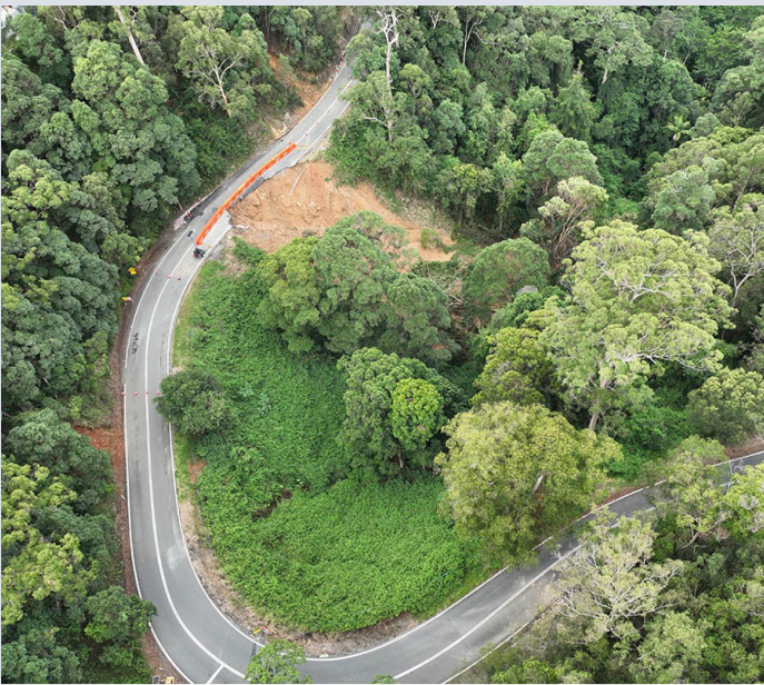
Beechmont Road – embankment failure (late March 2022)
