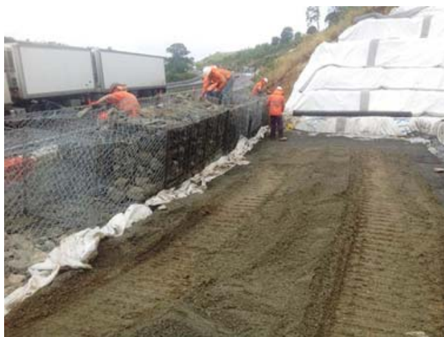
Above: works underway filling gabion baskets at One Tree Hill on the Warrego Highway - July 2014
