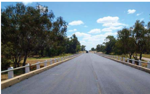
Completed section of the Landsborough Highway between Morven and Auguthella (top) and Barcoo River Bridge works 60km northwest of Tambo (bottom)
