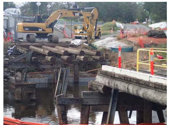
Right: stripping of the deck as part of the removal of the original Grigor timber bridge, March 2014
