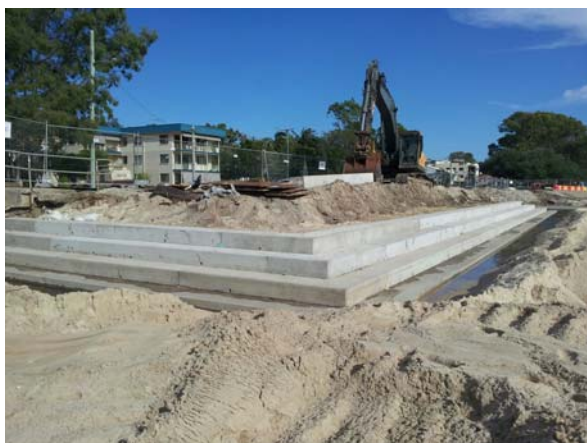
Right: Construction progress on the new stepped seawall, part of Stage one of the Bongaree Seawall - March 2014
