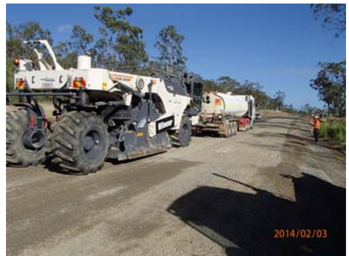
Above: stabilising works underway on the Bruce Highway (Benaraby to Rockhampton), south of Mt Larcom - February 2014
