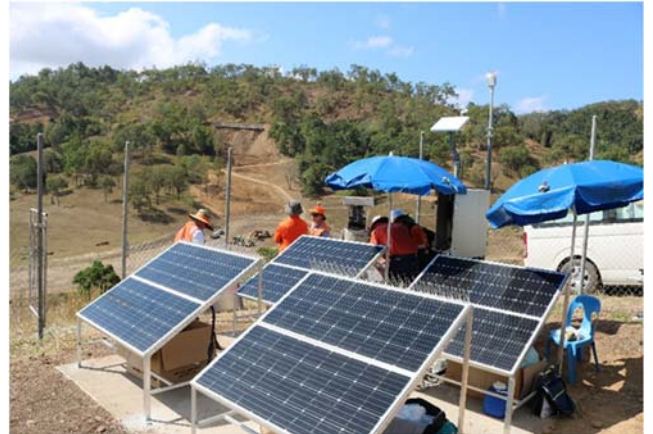
Monitoring station at Sarina Range main landslip site (above)
