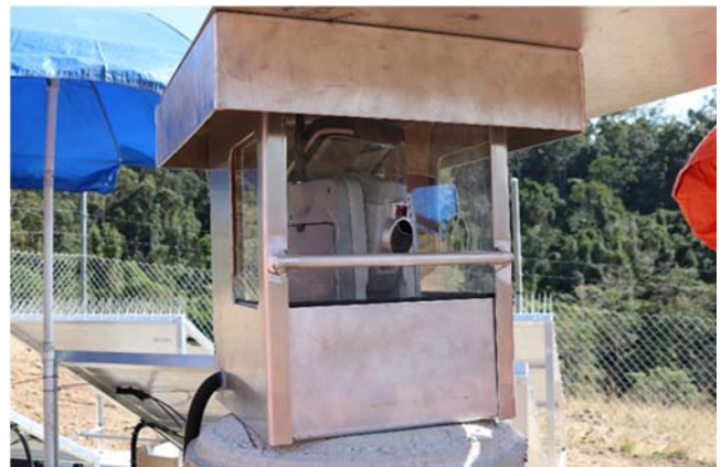
Sensor installed upslope to monitor movement (above)
