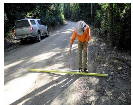
Above: Damage to Black Mountain Road, May 2011
