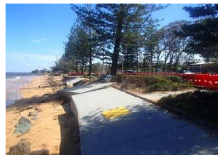
Above: Damage to Margate Parade seawall
