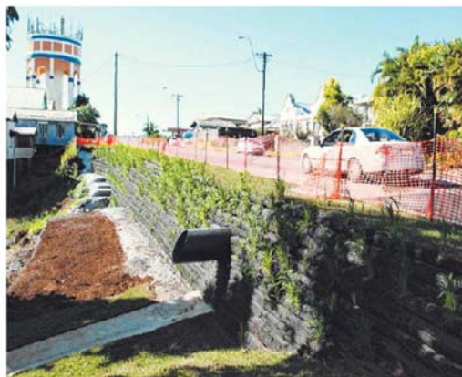
REPAIRED: A retaining wall has been built below Mourilyan Road in Innisfail as part of a landslip stabilisation project in the wake of Cyclone Yasi. Picture: Supplied
