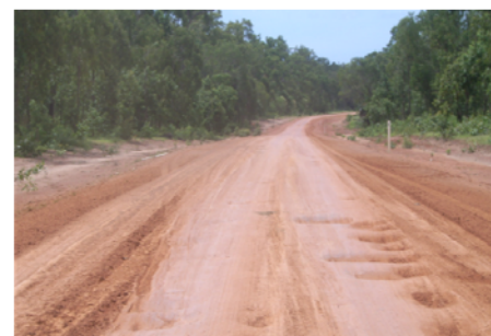
Above: Damage to Weipa-Mapoon Access Road
