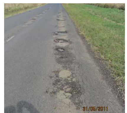
Above: Damage to Roadvale Harrisville Road
