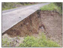
A landslide which is part of the works to be done on the Jimna Range
