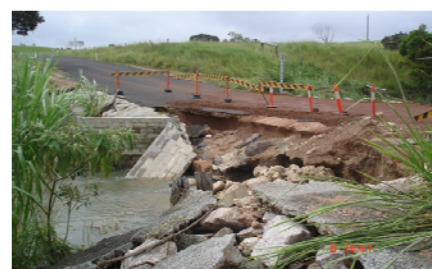
Above: Damage to Boar Pocket Road, Tablelands Regional Council
