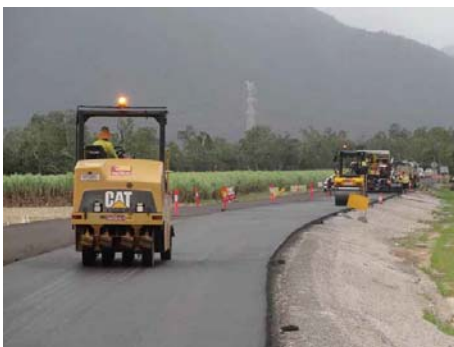
Above: asphalt overlay south of Seymour River Overflow Bridge, Bruce Highway (Ingham to Innisfail)
