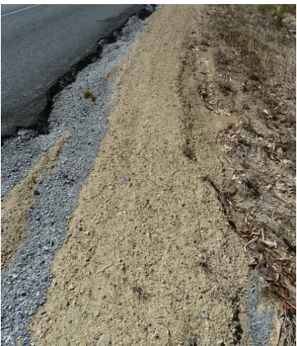
Left: Damage to Round Hill Road
