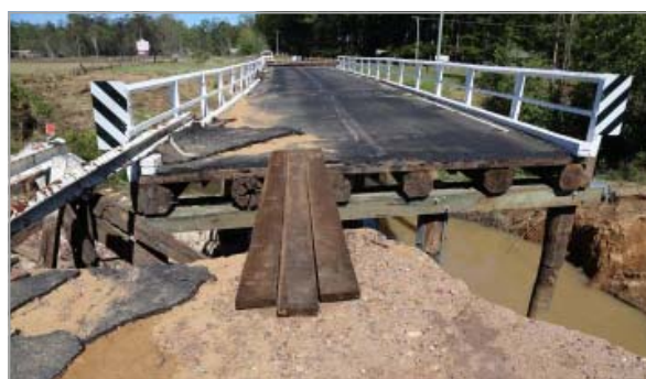
Above: damage to Clifton Creek Bridge (Brooweena), Fraser Coast
