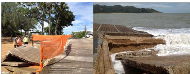
Above: showing damage to Horseshoe Bay boat ramp, Magnetic Island.
