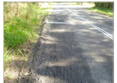
Above: showing damage to sections of Traveston Road.
