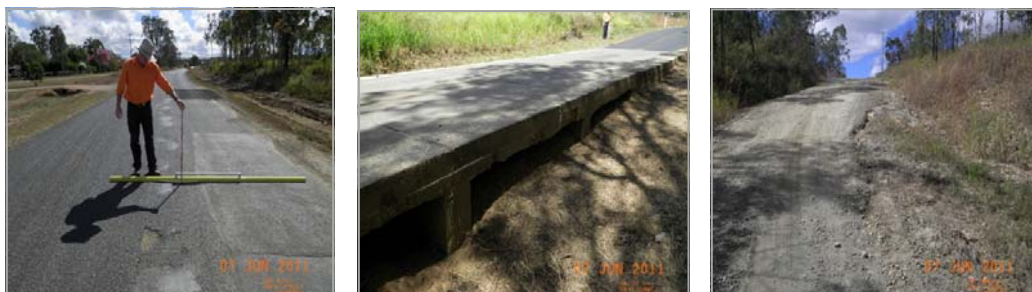
Above: damage to sections of Bilwon Road.
