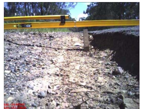
Above: showing damage to Bucca Road following 2013 flooding
