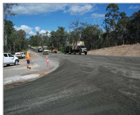
Above: Bruce Highway (Gin Gin to Benaraby) granular overlay in progress prior to cement modification.
