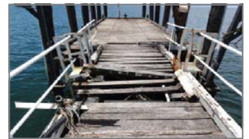
Above: damaged Clump Point jetty.
