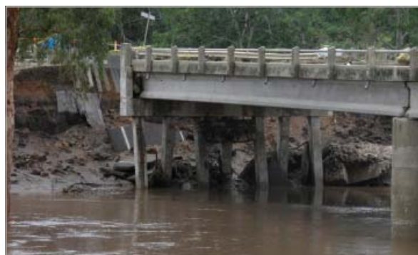
Above: Scouring damage at bridge abutments, Neerkol Creek, west of Rockhampton
