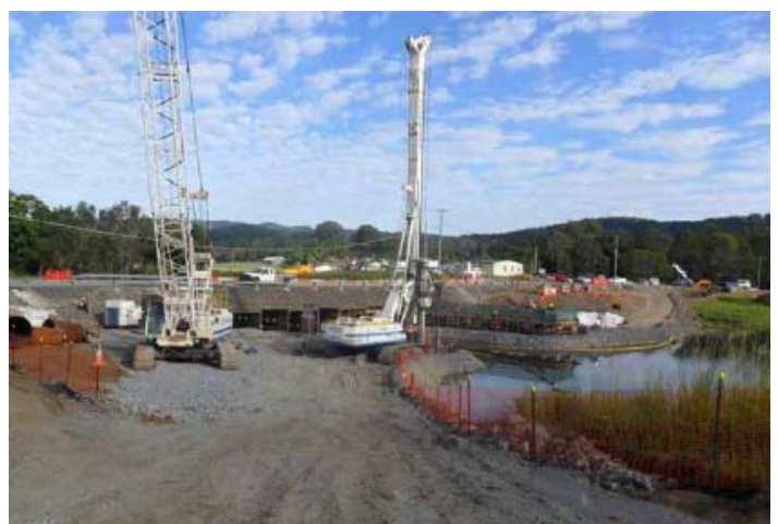
Above: Piling on the east bank of John Muntz Bridge - Tamborine Oxenford Road, May 2013.
