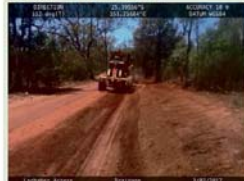
Lochaber Access Rd, Eidsvold 'under construction'. Council acknowledges the Natural Disaster Relief and Recovery Arrangements (NDRRA) funding is a joint Commonwealth and State Government program.
