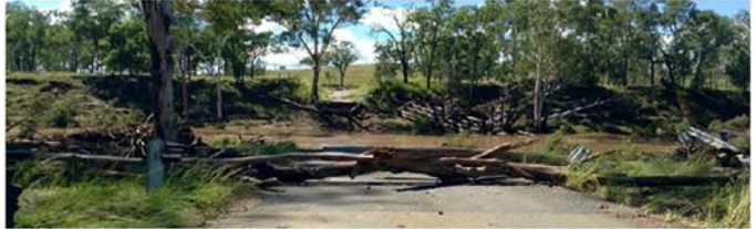
Works progressing on the Burnett River Bridge washed away during Cyclone Marcia
