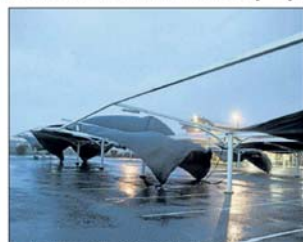
In Mackay's Northern Beaches shade sails were destroyed, with chains left flying in the strong winds.
