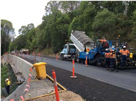
Asphalting works underway on Kin Kin Road in January 2015 - one of the last 2013 event works completed by DTMR
