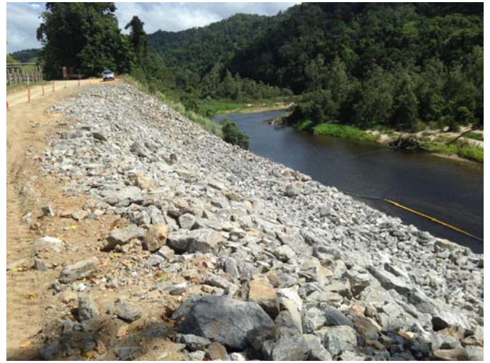
Landslip stabilisation work completed on Upper Daintree Road, adjacent to the Daintree River.
