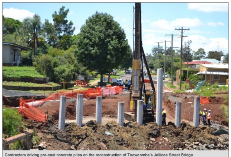
Contractors driving pre-cast concrete piles on the reconstruction of Toowoomba's Jellicoe Street Bridge
