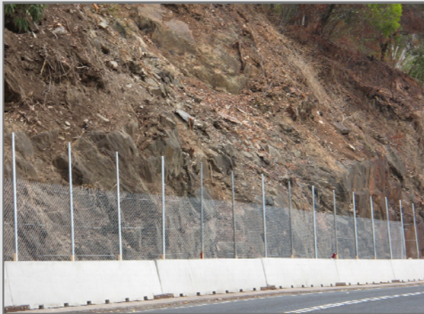
Above: Damage to a slope above the Captain Cook Highway, between Cairns and Mossman
