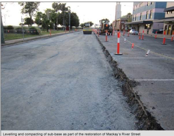
Levelling and compacting of sub-base as part of the restoration of Mackay's River Street
