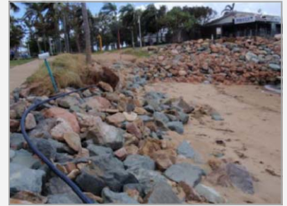
Above: Damage to rock wall at Gregory St on The Strand.
