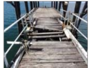
Above: damaged jetty at Clump Point
