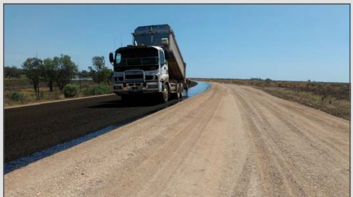
Above: Bitumen sealing works on the Castlereagh Highway, 7km outside of St George, November 2012.
