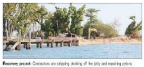
Recovery project: Contractors are stripping decking of the jetties and housing pylons
