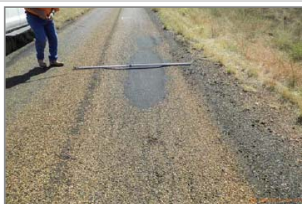
Right: Major pavement deformation from heavy traffic following the Monsoonal flood event.
