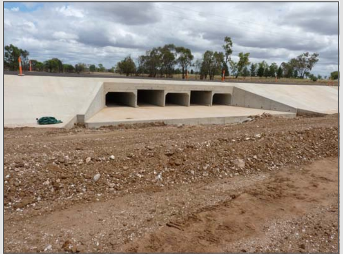
Above: Replaced culvert on the Castlereagh Highway between Kurray Station Airfield and Doondi Station, October 2012
