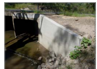
Images above showing damage to the culvert on Callandoon Road
