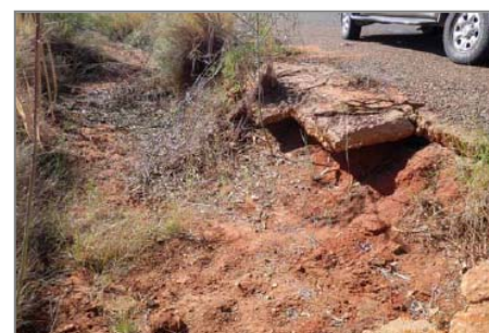
Above: Damage to concrete batter on Diamantina Developmental Road
