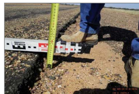
Above: Showing scouring to the road shoulder.
