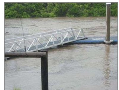
Images above: Balgal Beach Pontoon destroyed - February 2011
