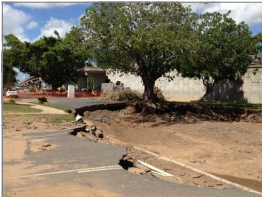
Above: Severely damaged Don Tallon Bridge in Bundaberg following the floods
