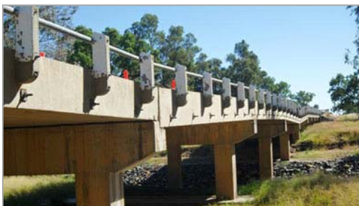
Above: Damage to the bridge structure— June 2012
