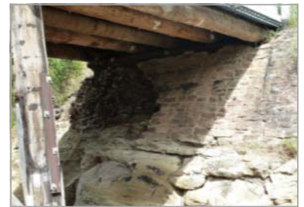
Above: Damage to Djuan Road Bridge from 2011 flood events weather permitting
