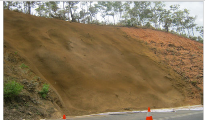
Above: Slope stabilisation works—a section of the embankment above the road treated with shotcrete.
