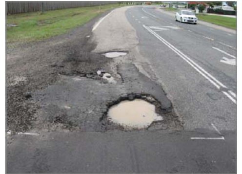
Above: Damage to Bruce Highway near Bowen following the 2010/11 wet weather event
