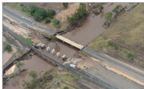
Above: Damage to Capricorn Highway at Neerkol Creek (Courtesy www.themorningbulletin.com.au ).
