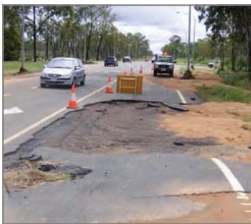
Peak Downs Highway – showing damage as a result of the 2010-11 events.
