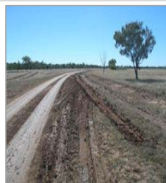
Above: image showing loss of gravel
