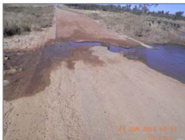
Above: Damage to Narounyah Road from 2012 floods
