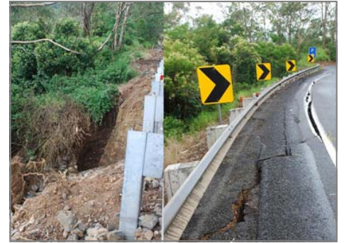
Above: Damage to slopes and pavement on the Toowoomba Range crossing, Warrego Highway
