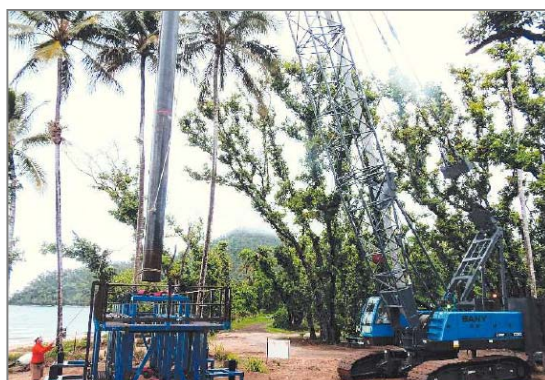
Left: Pile-driving works on Dunk Island for the new jetty. The equipment will be moved to the mainland to start the new Clump Point jetty. (Courtesy: General News, 13 February 2013)
