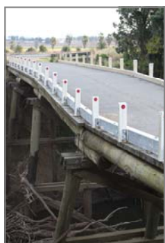
Above: damage to Stokes Bridge
