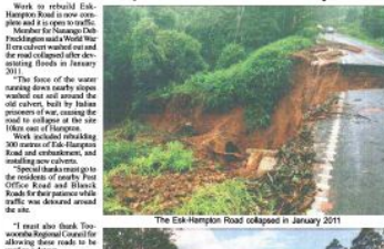
The Esk-Hampton Road collapsed in January 2011.
