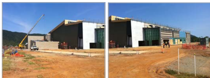
Above: Progress of construction of the Cairns Cyclone Shelter - Edmonton Leisure Centre.
